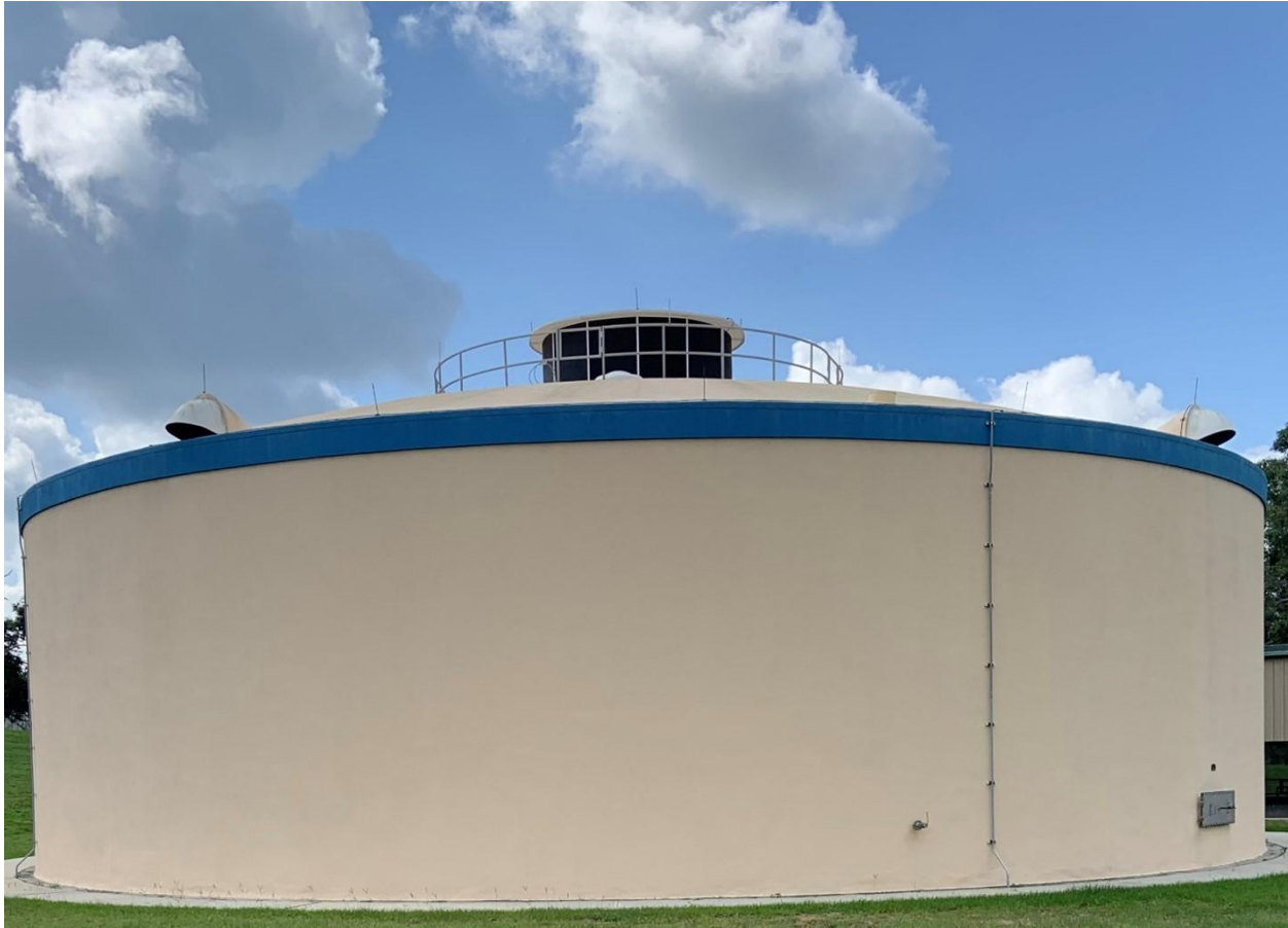
Figure 1 Cherry Hill Water Treatment Facility.
