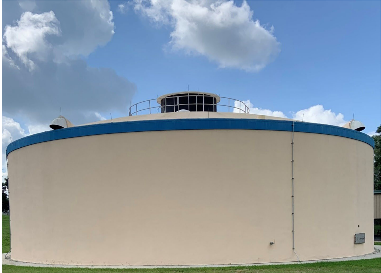
Figure 1 Cherry Hill Water Treatment Facility.
